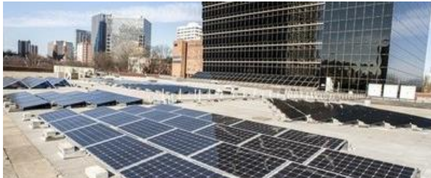
50 kW-1MW, Commercial Building
